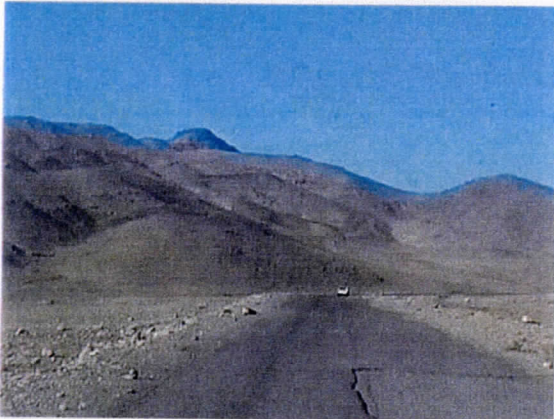
photo 9. Typical view of the route as it approaches the pass into the Bagram Valley. The road is constructed of asphalt concrete approximately 10m wide.
